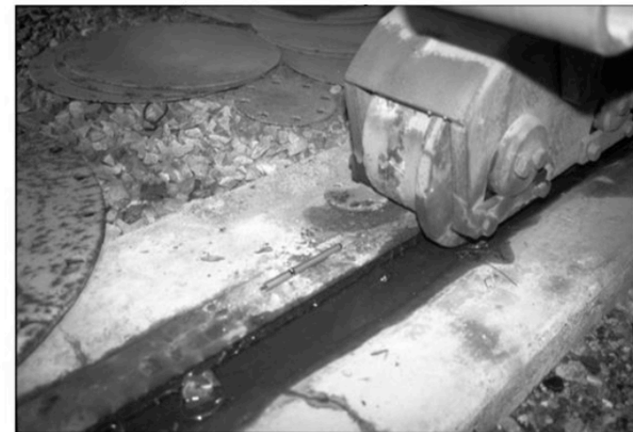
Izmit, 1999, derailment of wheels
